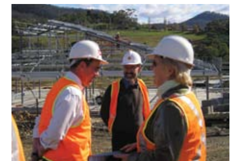
The Hon. Judy Jackson MHA, Minister for Justice and Industrial Relations, announces the additional nine million dollar funding boost for the Prisons Infrastructure Redevelopment Program
