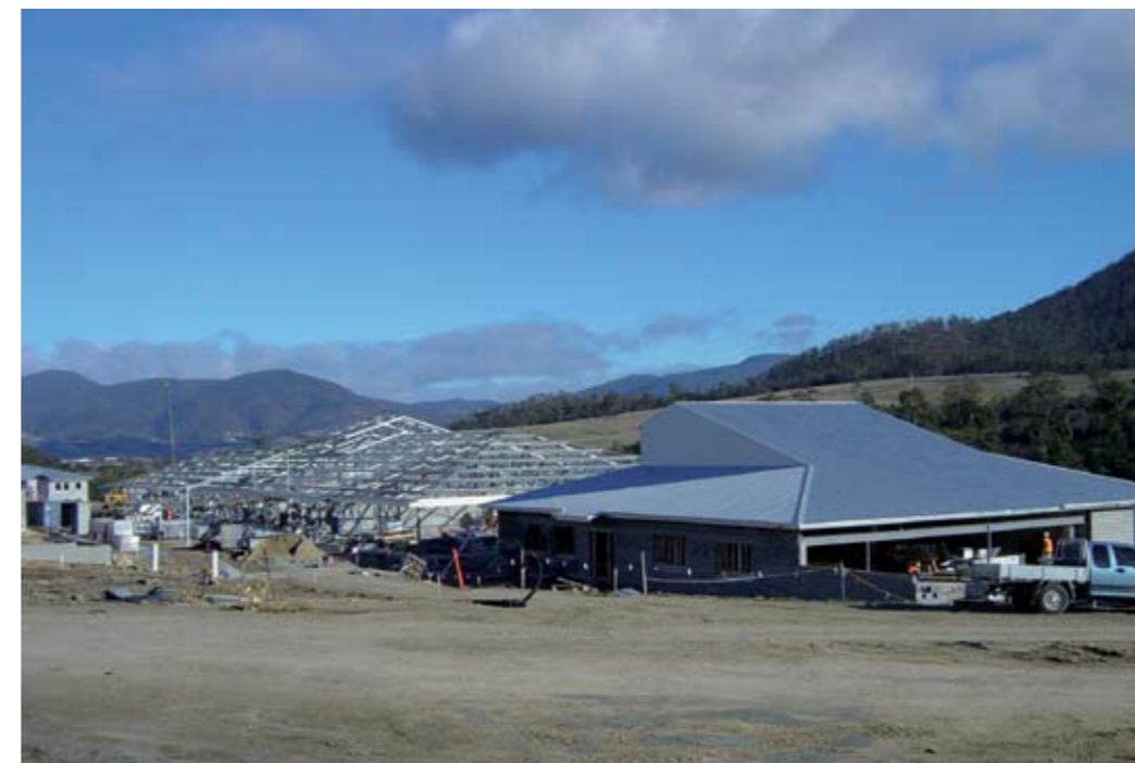
Below: Steelworks for central facilities block (left) and new visits building (right)
