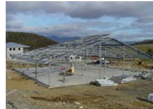
New education building under construction with medium security cell block at left
